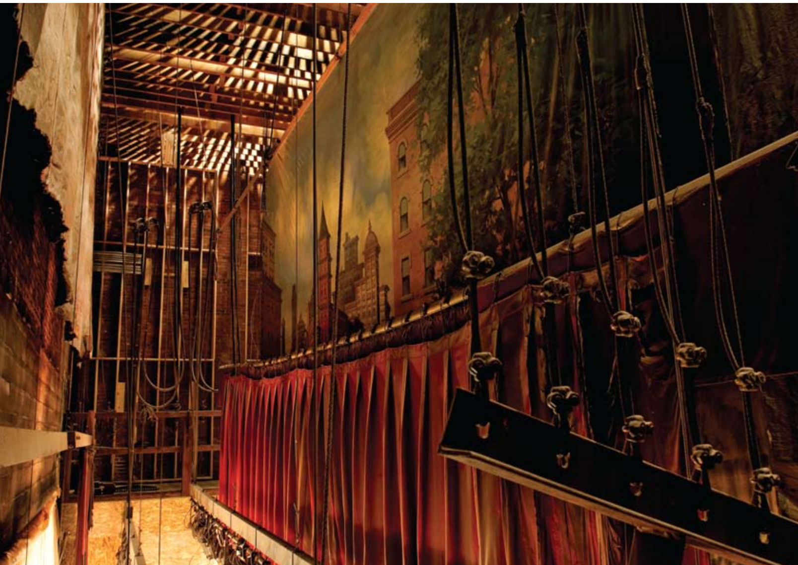
The fireproof curtain between the auditorium and the stage helped stop the 2006 fire from burning the back stage area and the five original 1921 backdrops that were part of the Twin City Scenic Company Collection. There are still tomato seeds stuck to one of the backdrops left over from vaudeville days.
